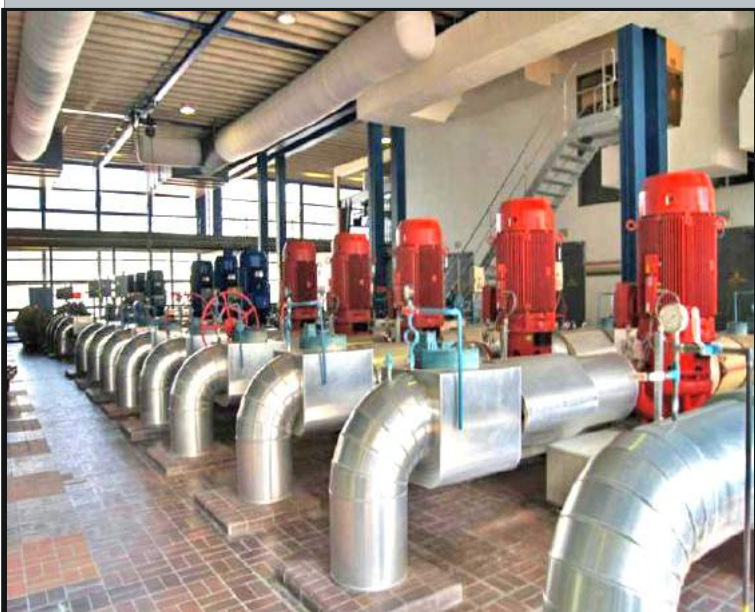
IN-LINE PUMPS WORKING AT A.C PLANTS
